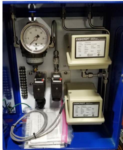
BTM Control Box (as built)
