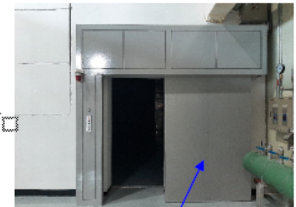
Sliding shielding door
