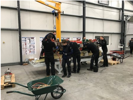
Quadrupole / sextupole girder
