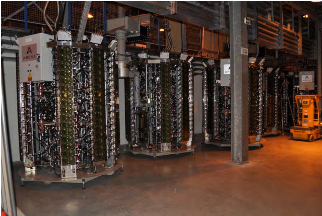
Figure 5.15: Three 150 kW – 352 MHz SSAs in cell 23 of the existing storage ring – ELTA-AREVA / SOLEIL design.
