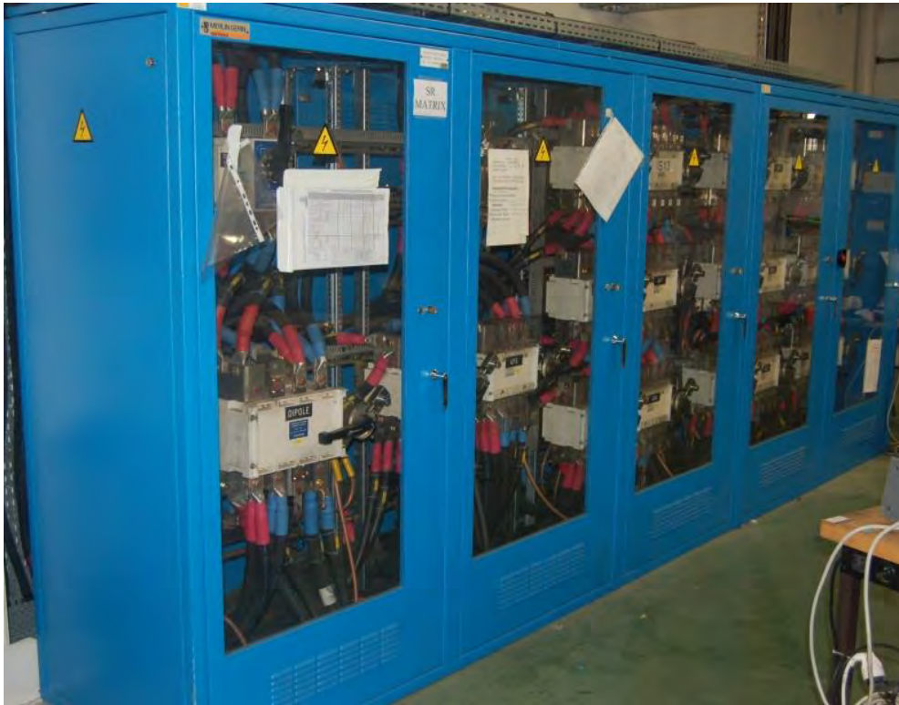
Figure 4.7: Switching Matrix serving the family power supplies.
