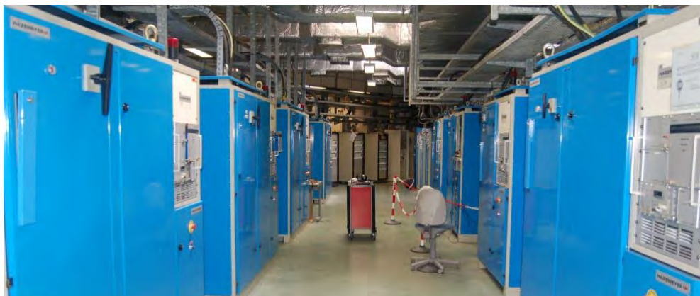
Figure 4.6: SRDC room with future refurbished AC/DC rectifiers.
